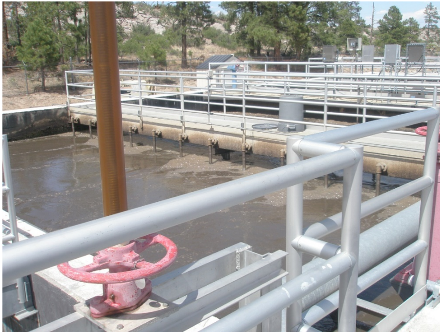
Photograph - NPDES-13S-18-0011 SWWS Equalization Basins
