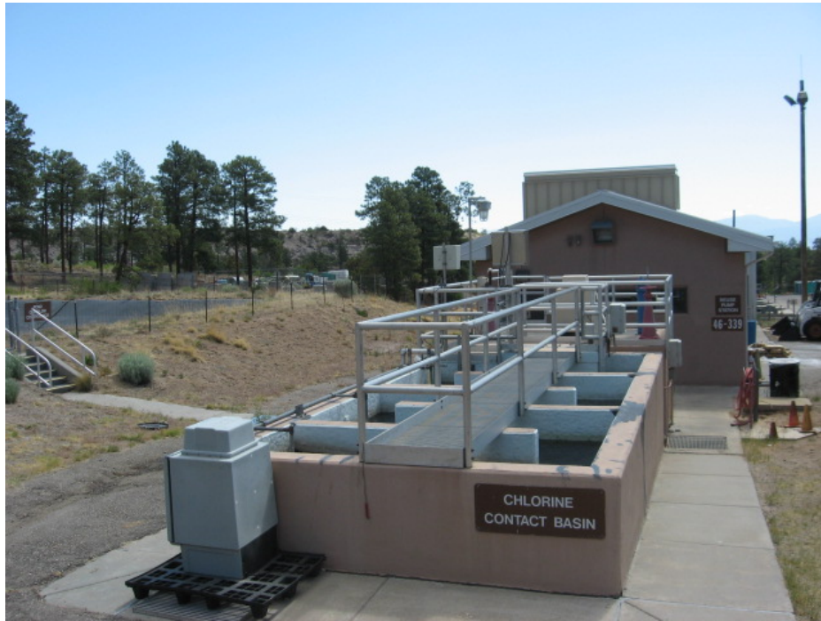
Photograph - NPDES-13S-18-014 SWWS Chlorine Contact Chamber
