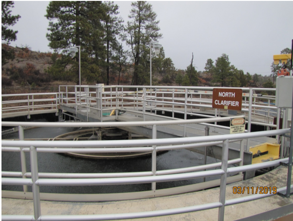
Photograph - NPDES-13S-18-013 SWWS Clarifier
