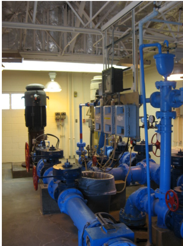
Photograph - NPDES-13S-18-018 SWWS Reuse Pumps and Chlorine Analyzer
