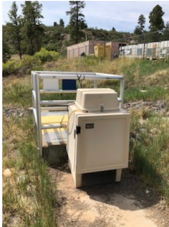
Photograph - NPDES-13S-18-005 Outfall 13S Ability to Collect Representative Compliance Samples at the Outfall
