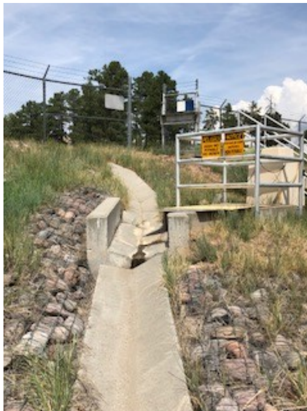
Photograph - NPDES-13S-18-002 Outfall 13S Condition
