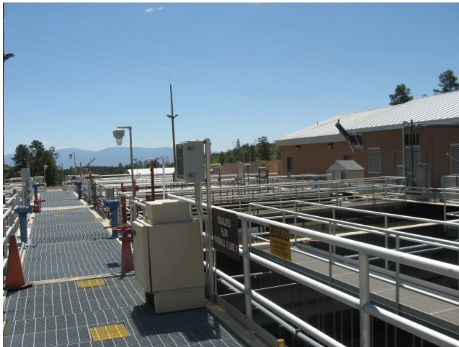
Photograph - NPDES-13S-18-0012 SWWS Aeration Basins
