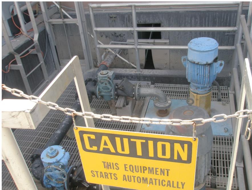
Photograph - NPDES-13S-18-008 SWWS Grit Chamber
