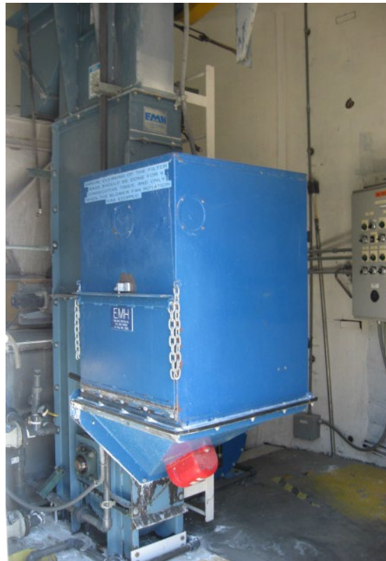
Photograph - NPDES-13S-18-0010 SWWS Soda Ash Feed System
