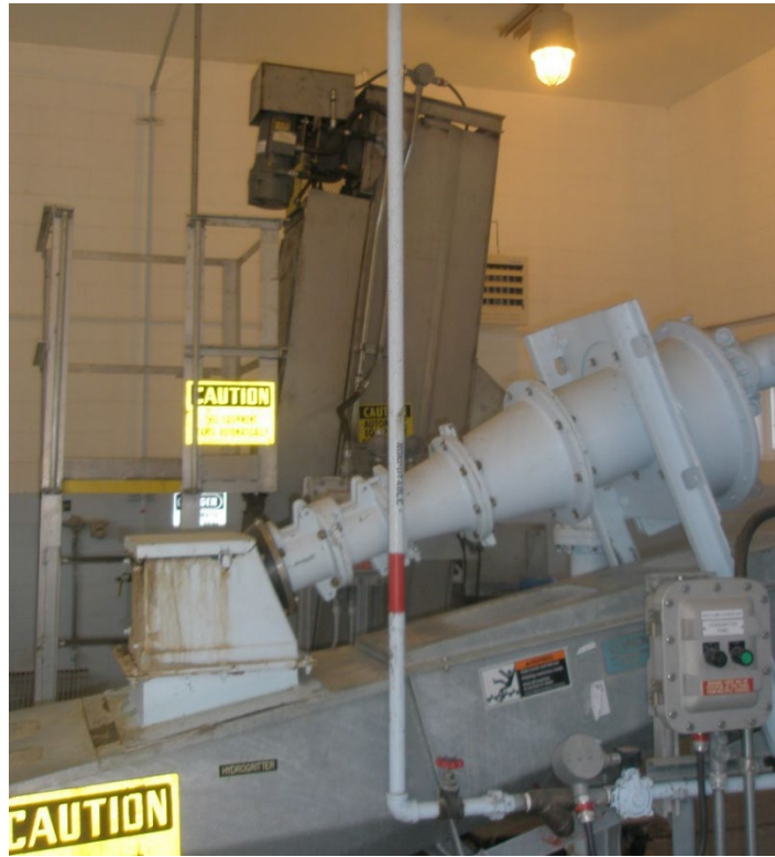
Photograph - NPDES-13S-18-007 SWWS Bar Screen at the Headworks
