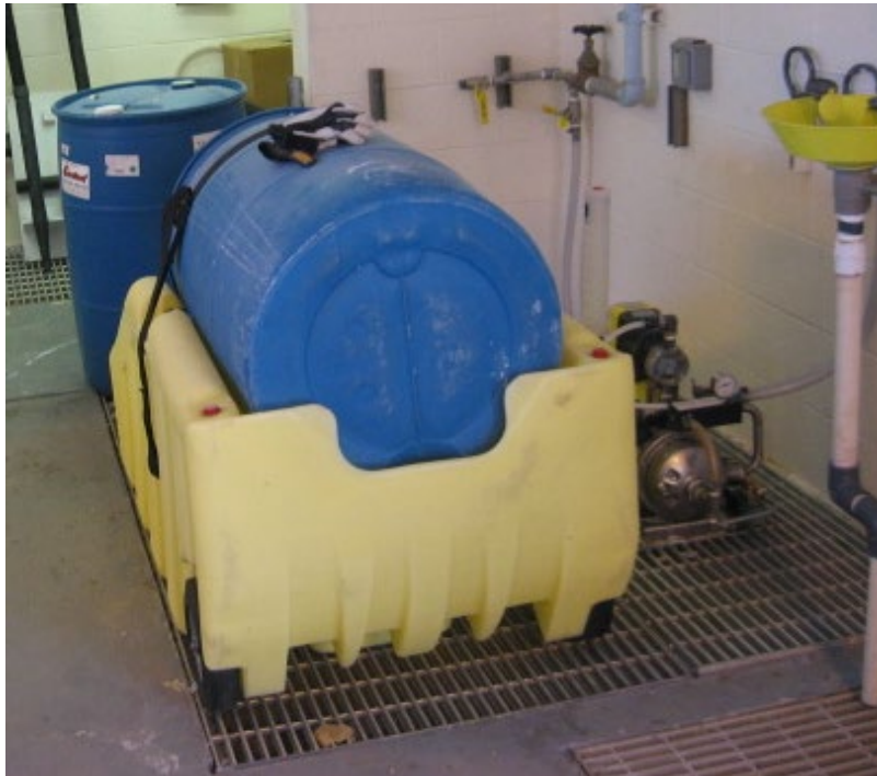
Photograph - NPDES-13S-18-016 SWWS Sludge Polymer Feed Tank
