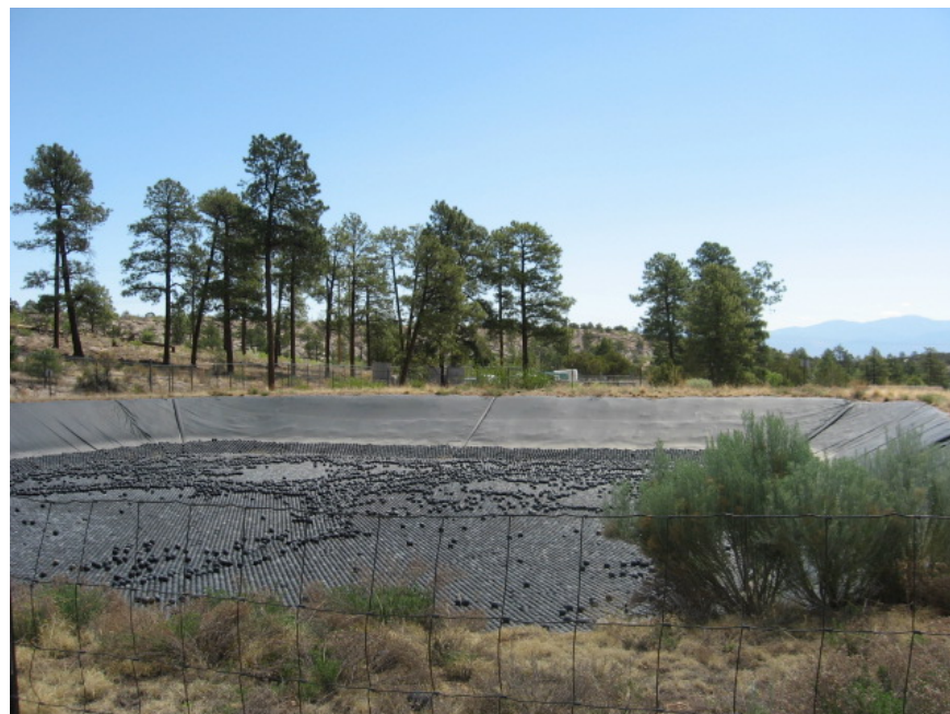
Photograph - NPDES-13S-18-017 SWWS Effluent Holding Pond
